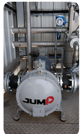
Pumping unit JE24s
